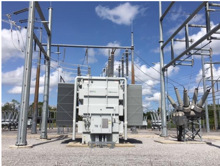
230kV/69kV Transformer Detail
