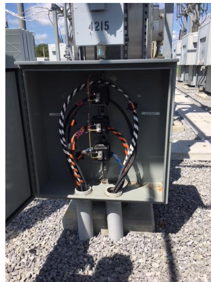
Internal wiring for CTs (E-frame)
