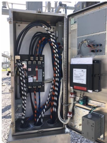
Internal wiring for ATS (E-Frame)
