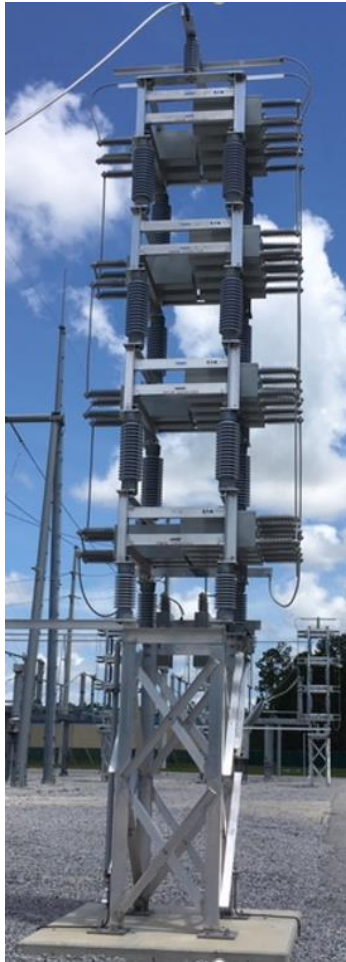
245KV CAPACITOR BANK
