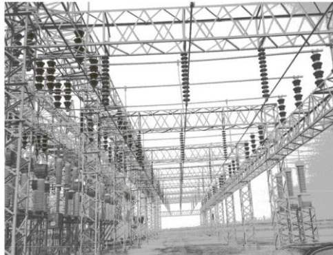
Suspension Insulators in a High Profile Substation
