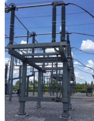
230KV GROUP OPERATED SWITCH
