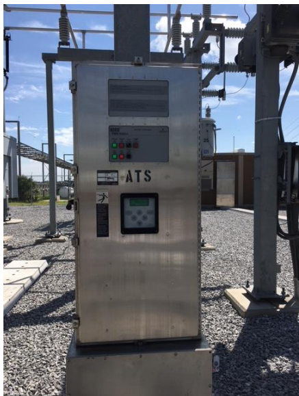
External view of ATS (E-Frame)
