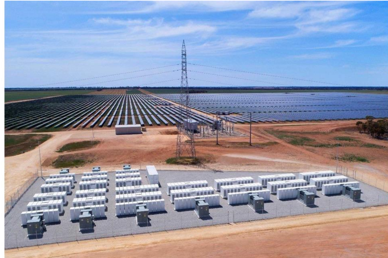
50 MWh Tesla Battery at a Solar Farm In Australia
