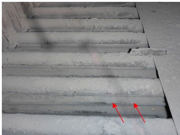
Buildup between tubes
