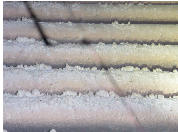
Scale buildup on tubes
