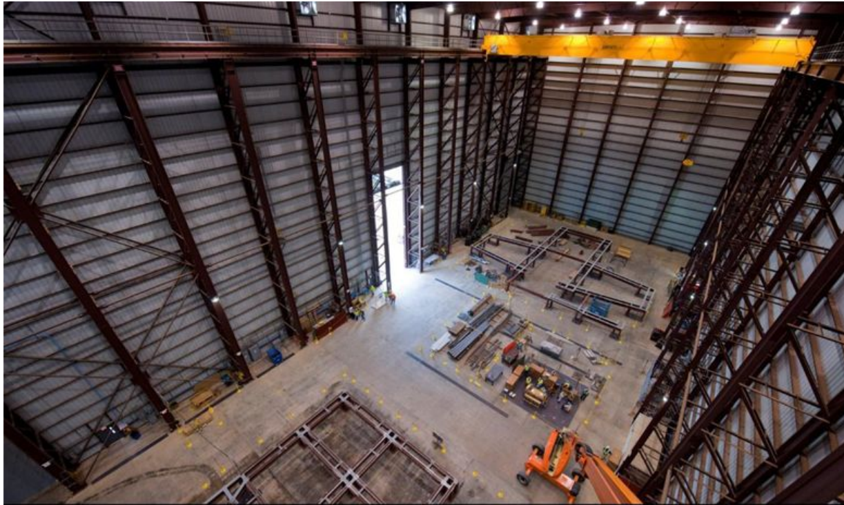
Inside the Plant Vogtle 3 and 4 module assembly building; two frames in place for use in assembling large structural modules. September 21, 2011
