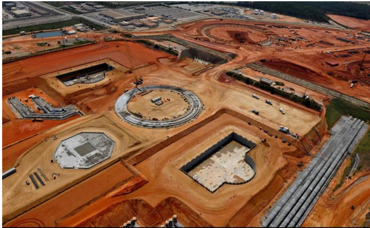
Aerial photograph of Vogtle 3 and 4 construction site. Unit 3 is located at left and top of photo and Unit 4 to the right and bottom. Heavy lift derrick crane foundation in center. August 11, 2011 © 2011 Southern Company, Inc. All rights reserved.
