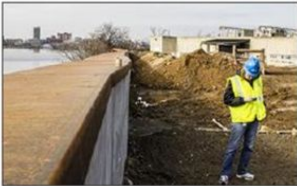
DC Water Flood Wall Source: Umair Irfan, eeneews.net
