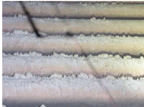
Scale buildup on tubes
