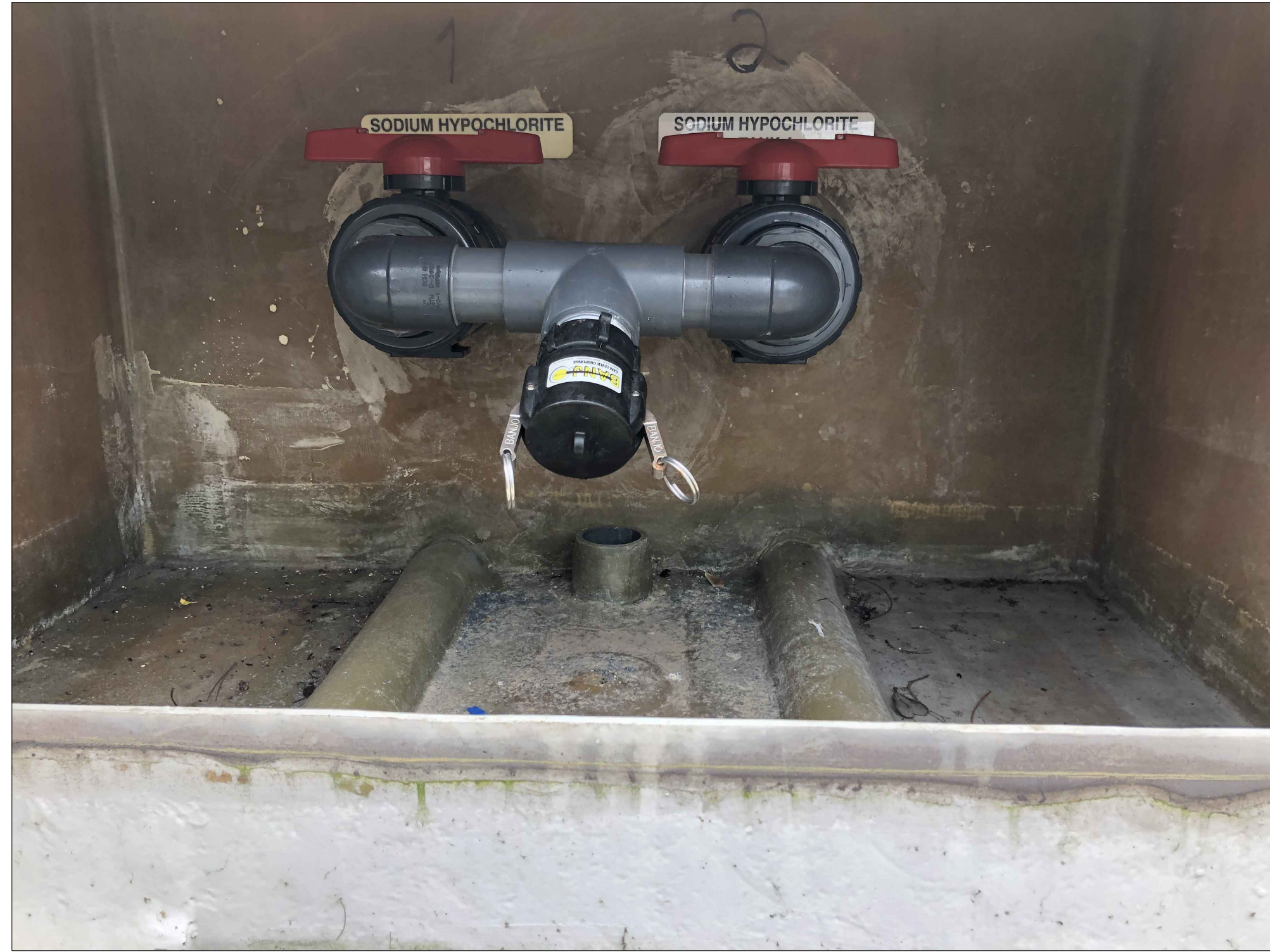
CHEMICAL FILL STATION PIPING
