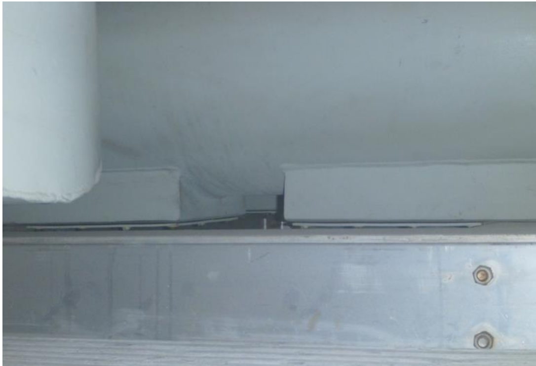
Five hard to access insulators.
