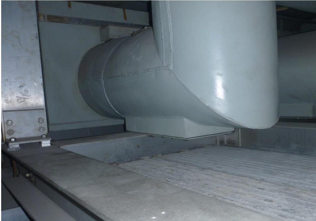
Five hard to access insulators.
