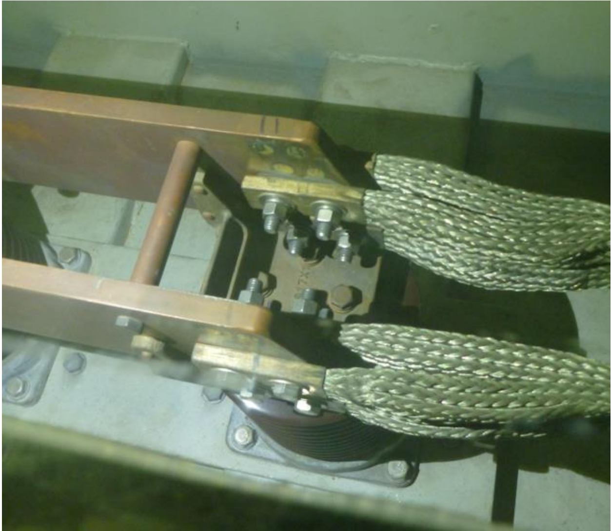
Middle of abandoned switch.
