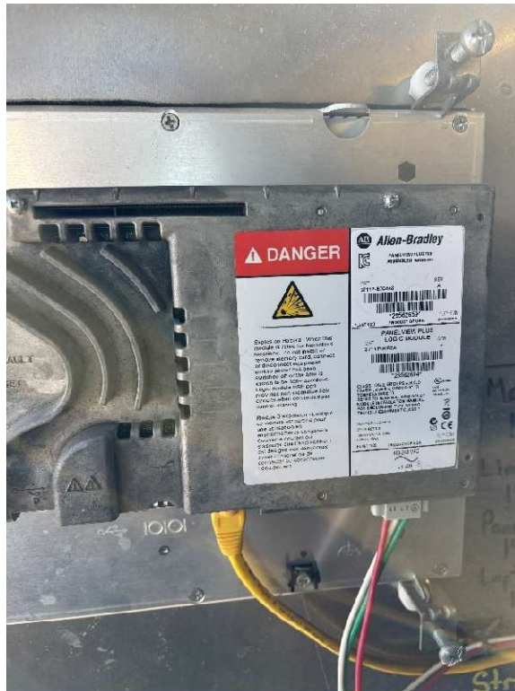
Figure 4: Existing Main CWTS PanelView 7 HMI
