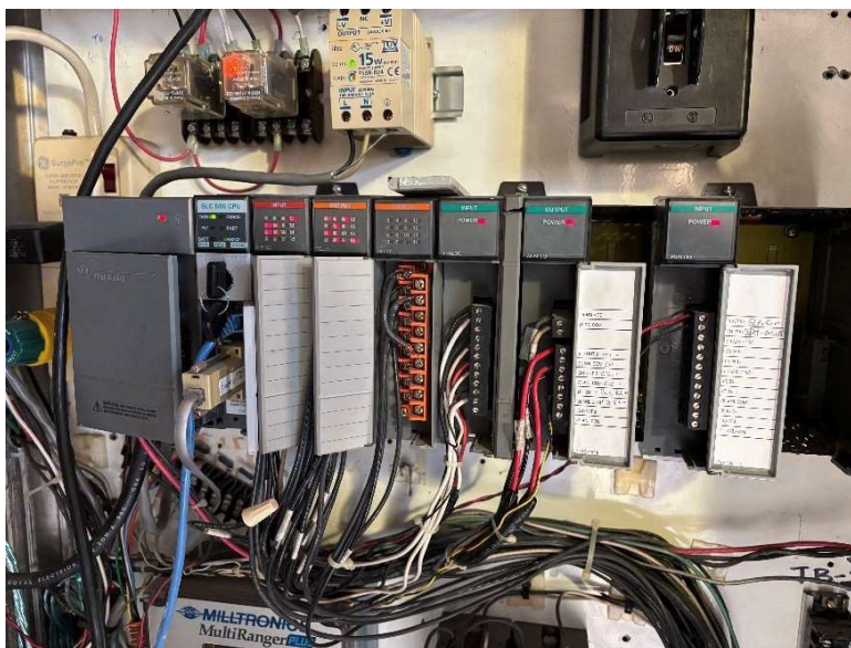
Figure 2: Existing LimeFeed SLC 5/05 Controller
