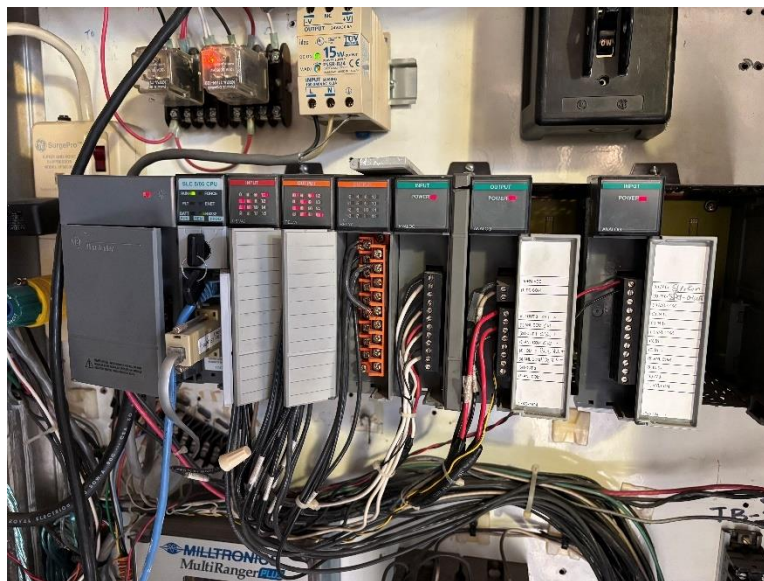
Figure 2: Existing LimeFeed SLC 5/05 Controller
