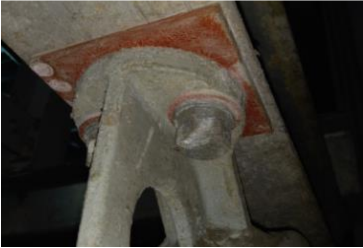
Figure 10. Twelve bolts per phase at each location.
