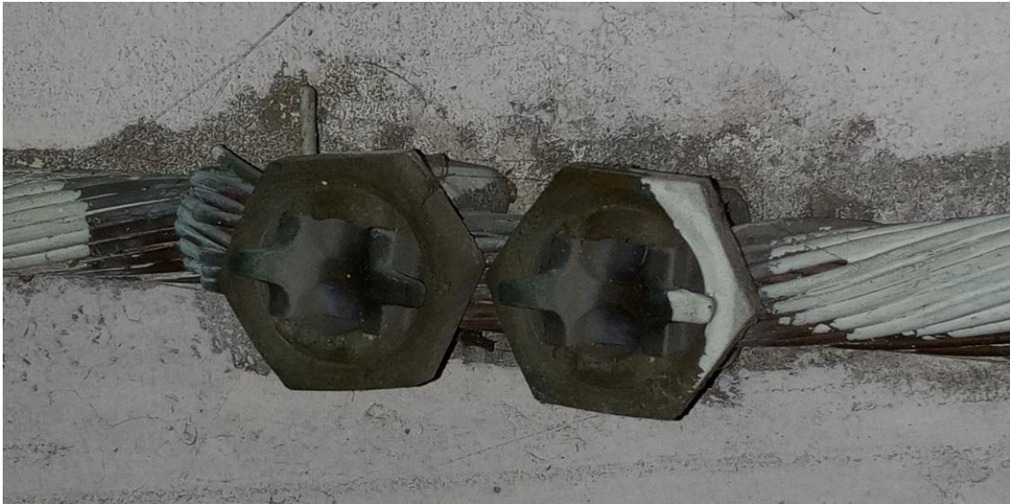
View of 500MCM on the Mezzanine.
