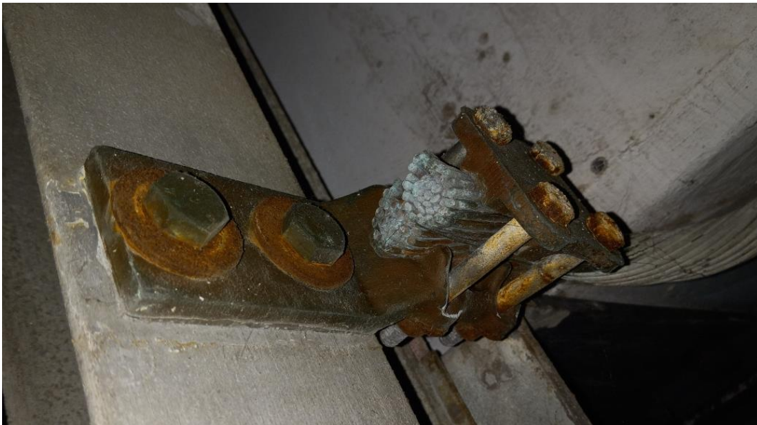
View of Bonding connection between Aluminum bus and cable.
