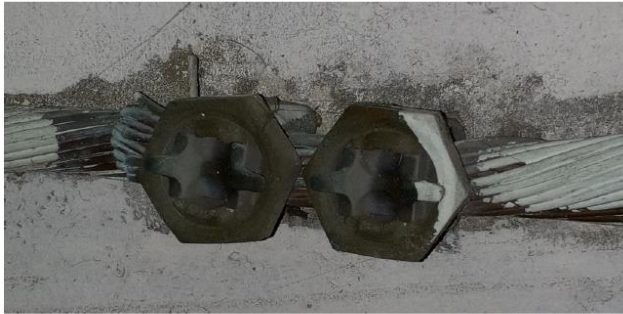
View of 500MCM on the Mezzanine.
