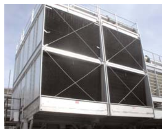
Picture 2 - Cooling Tower - Moly free is the way to be!
