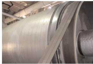
Picture 1 - Biosolids Pellets Drying Drum
